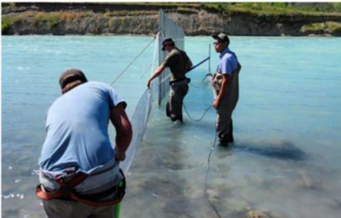
TNG Fisheries crew worked with technical partners from EcoFish Research Ltd. to install a new fish passage SONAR upstream of the slide at Hanceville on (Aug 8)
